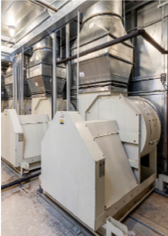
LABORATORY EXHAUST FANS
